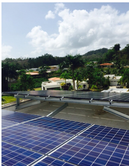
Solar carports at Cooperativa Jesús Obrero's Guaynabo location provide electricity for the building.
